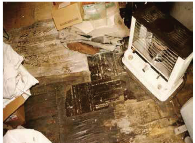
Vinyl Floor Tiles and Adhesive Mastic (on wood floor, damaged 9" X 9" tiles)
