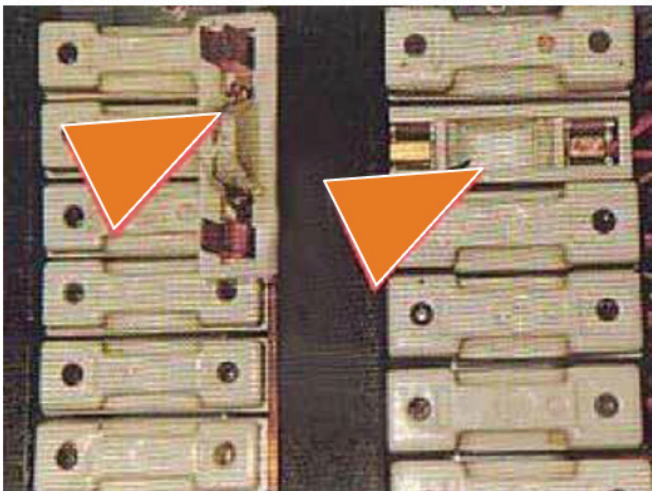
Asbestos Rope (electrical fuse board)
