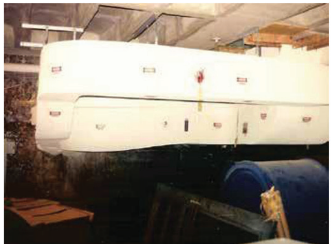
Heating and Cooling Duct Insulation (HVAC)
