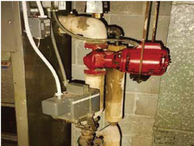
Fire Sprinkler Pump Piping Insulation
