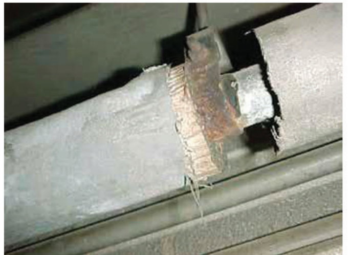
Pipe Insulation (damaged)
