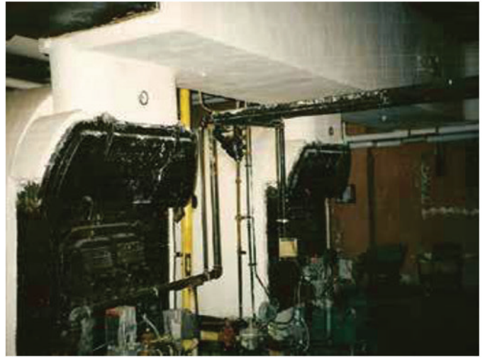
Boiler and Pipe Insulation
