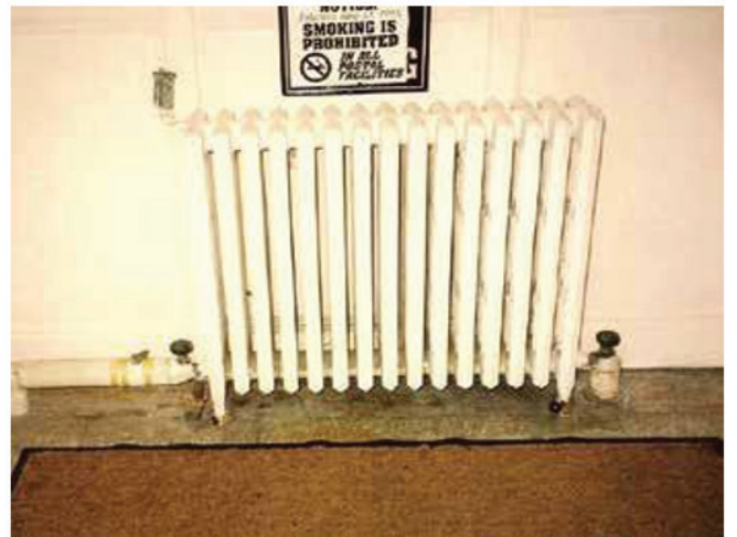
Radiator (insulation on piping and valves)
