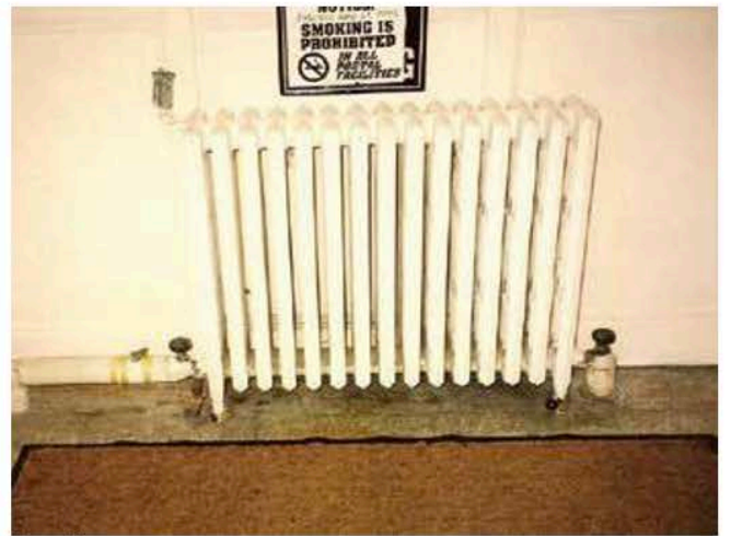
Radiator (insulation on piping and valves)
