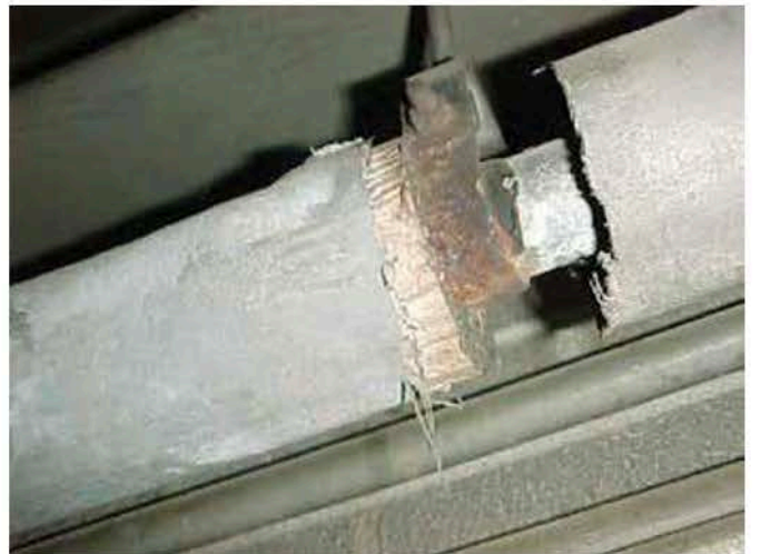
Pipe Insulation (damaged)
