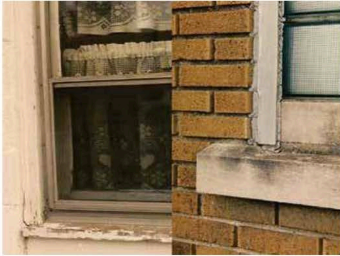
Window Glazing and Building Caulking (edges of glass panes and window frame)
