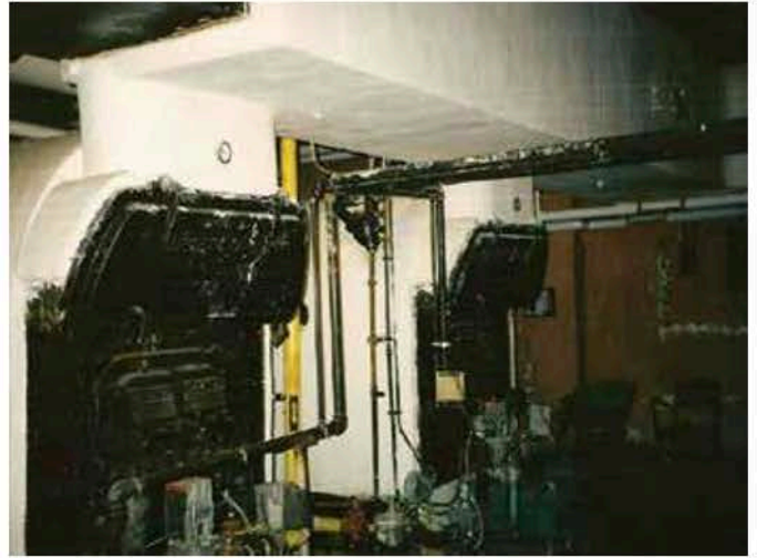
Boiler and Pipe Insulation
