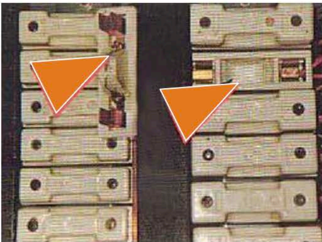
Asbestos Rope (electrical fuse board)
