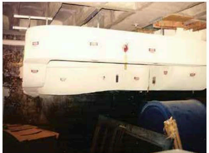
Heating and Cooling Duct Insulation (HVAC)
