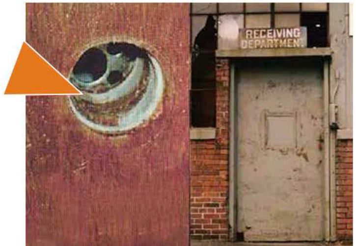
Fire Door (insulation inside door)
