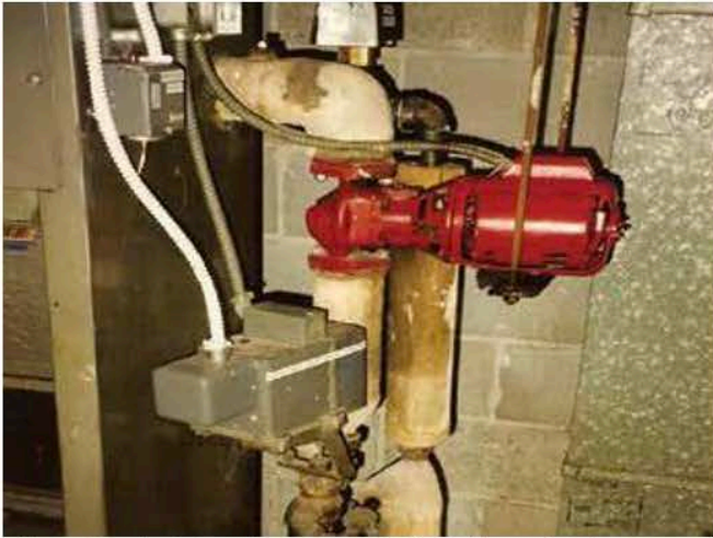
Fire Sprinkler Pump Piping Insulation
